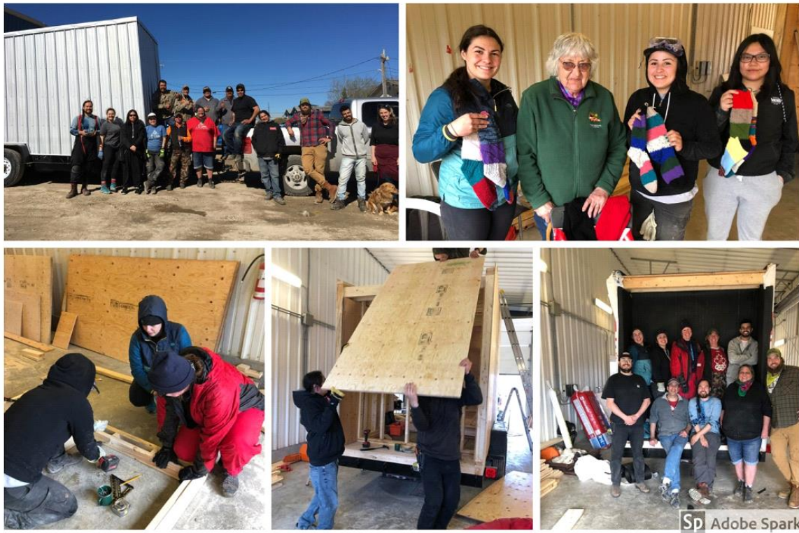
Photos from Left to right - 1,5 Happy team with the newly build structure; 3,4 Students are working to build the hut, 2 Gift sharing with a community elder.
